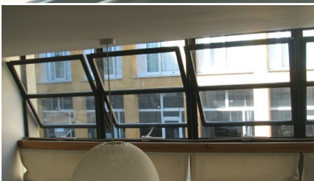
Manual Chains Fitted to a Bank of Centre Pivot Windows
